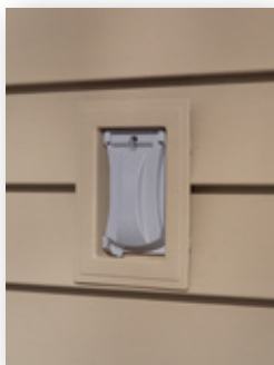
Recessed Electrical Blocks
