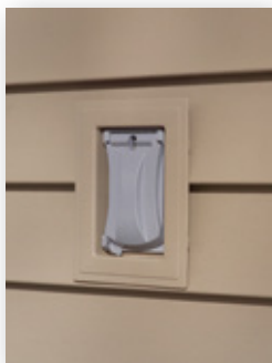
Recessed Electrical Blocks
