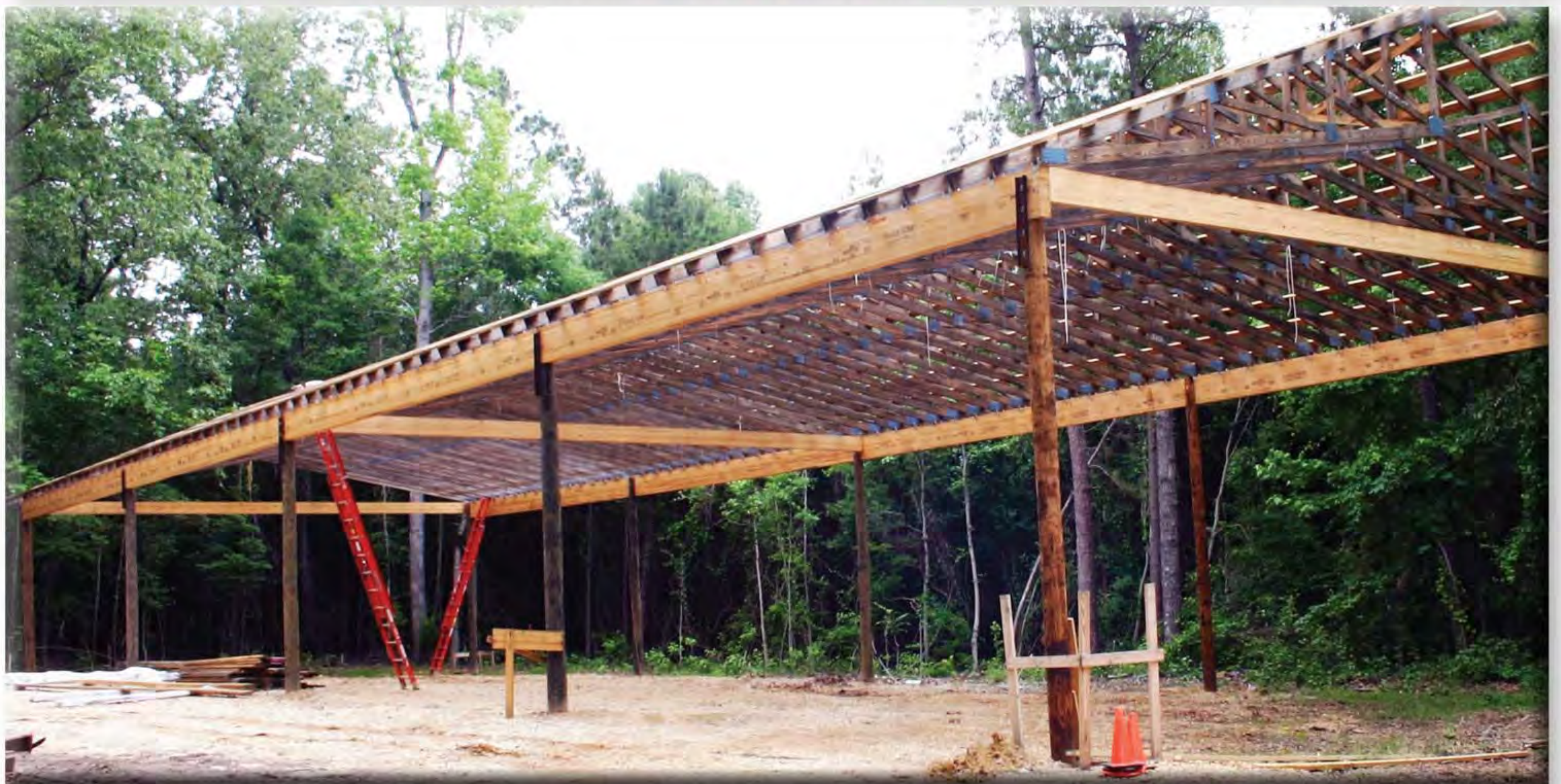
Above: New supply warehouse for Quality Electric Company in El Dorado, Arkansas
